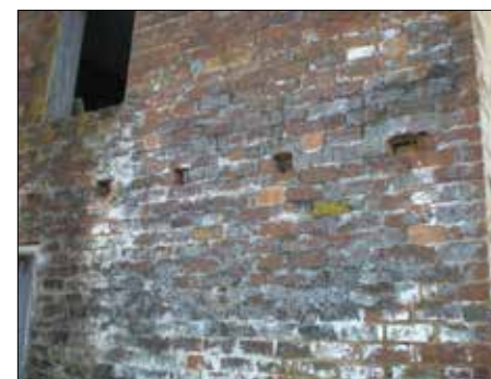
Pockets indicating where a porch was probably attached to the front.
